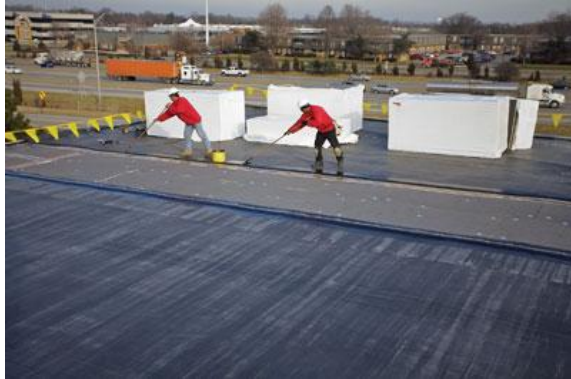
Workers install a Firestone RubberGard R.M.A. System, an EPDM roof. Firestone makes both EPDM and TPO roofs.
