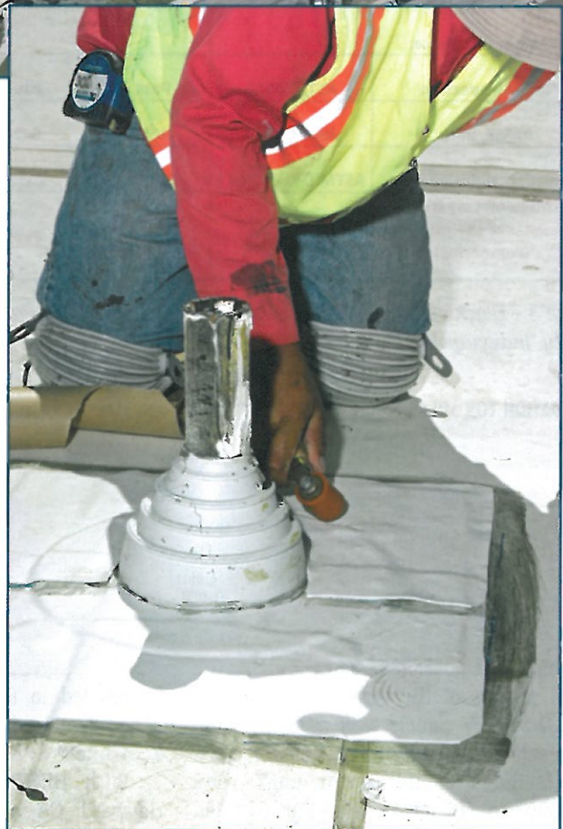
Photo 2 – Customized white EPDM target patches and boots used around the stanchions to support the PV panels helped expedite the installation process.
