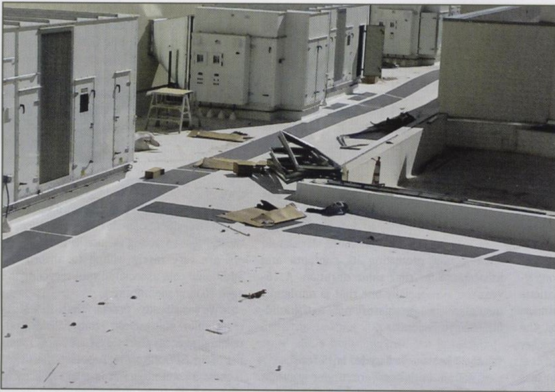
Figure 2 – Debris left by maintenance crews for various rooftop mechanical equipment increase the risk of a puncture.
