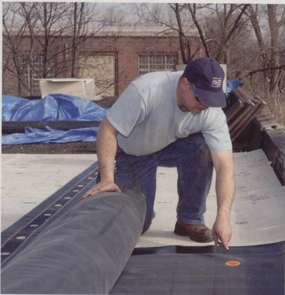
Restoring or recovering an existing roof system makes sense because the owner and environment receive numerous benefits besides a watertight roof, including extended service life, less waste generation, less ozone depletion, and little disturbance to building operations. (Photograph courtesy of Carlisle SynTec)
